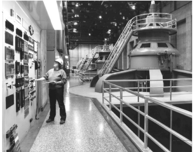
Roberta "Birdie" Hensley, Hoover Dam Powerplant Operator, makes adjustments to the Control Cubicle for Unit Number 1. Photo credit - Bureau of Reclamation.
