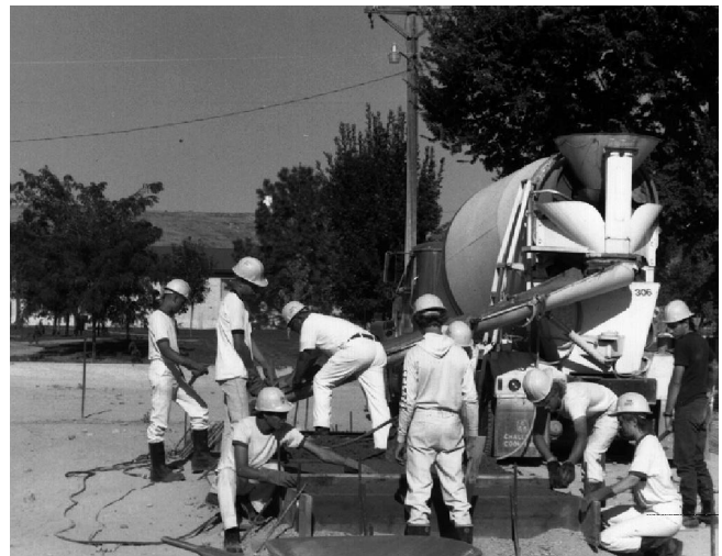
Reclamation's effort and attention in administering the Department of Labor's Job Corps Program has earned it the "Best Overall Operator" award over the past five years. This photo shows Job Corps students pouring cement for the first portion of a bridge to be built as a memorial at the Marsing, Idaho Job Corps Center.
