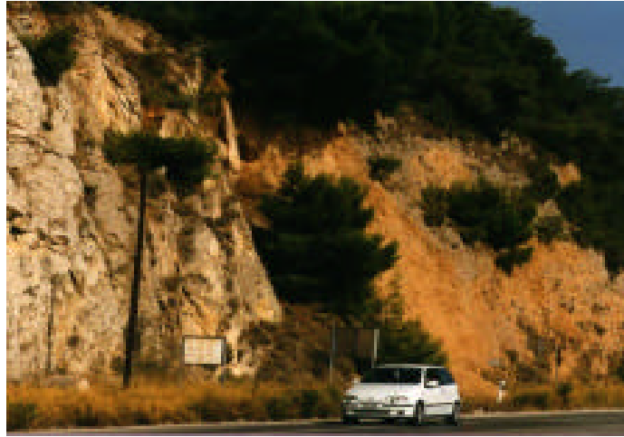
Figure 3. The Korinth fault is exposed in the roadcut along the highway between Kechries and Almiri, just to the west of Loutro Eleni. The fault, which intersects the road at the position of the front of the white car, juxtaposes limestone bedrock (left) against a thick sequence of consolidated colluvial sediments and interbedded red soils (right).
