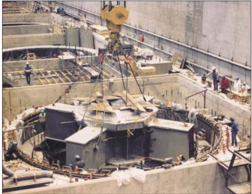
An upper generator bracket is installed in one of Limestone's turbine generators (units).
