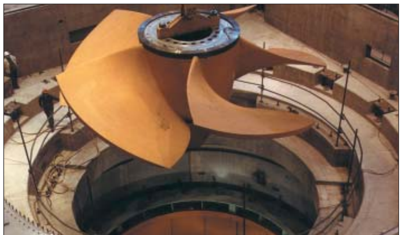
During construction, one of Long Spruce Generating Station's 98 MW turbine runners is prepared for placement.
