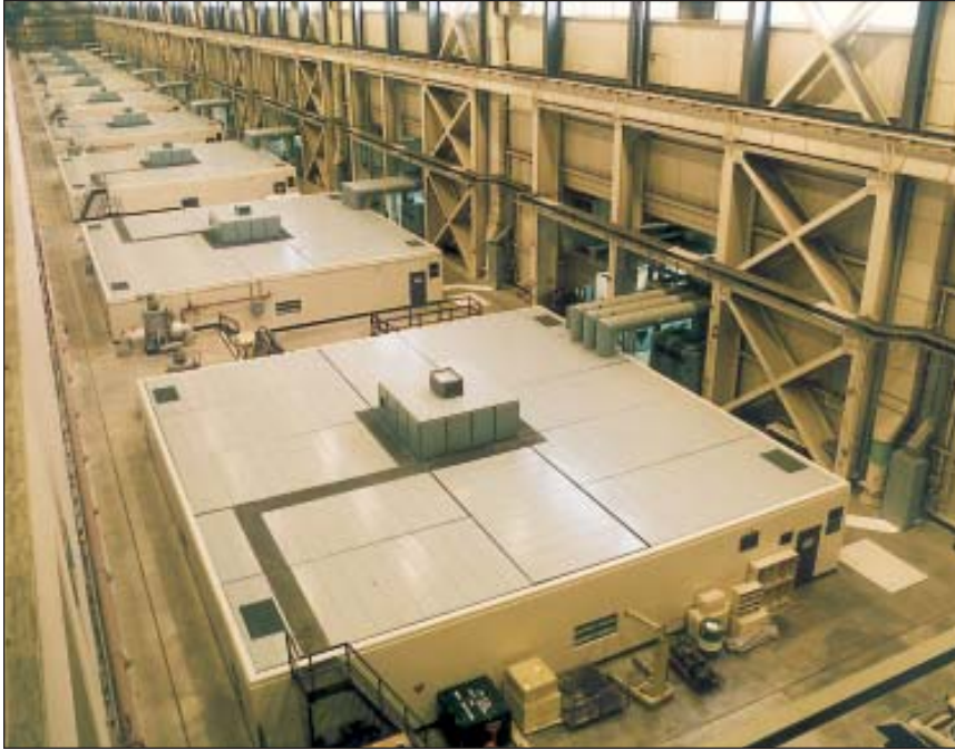
The interior of the powerhouse at Long Spruce Generating Station. Each of the square housings contains a turbine generator (called a unit). Canadian General Electric was the supplier of the 10 units.
