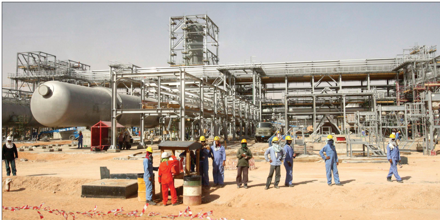
The Yokogawa process control system was selected for the Khurais central processing facility project in August 2006
