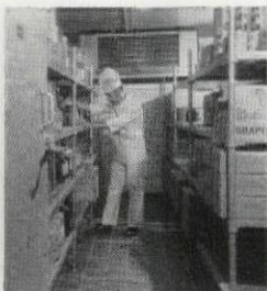
Low temp 'ED' electric defrost unit in walk-in cooler
