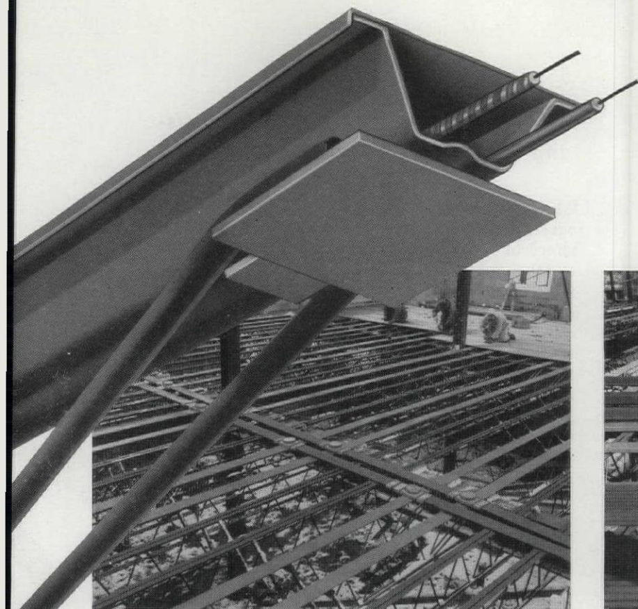
In this case, pairs of E/C Joists are alternated with pairs of standard joists at 18" o.c., and tie in with a two-duct system at 6'-0" o.c. The header ducts here were installed during a 4" snowfall, demonstrating that construction can proceed in bad weather.
