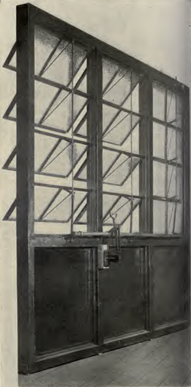
IRON AND WIRE GLASS WINDOW DETAIL—PENNSYLVANIA RAILROAD COMPANY'S NEW POWER HOUSE. Long Island City, N. Y. Westinghouse, Church, Kerr & Co., Engineers. The Hecla Iron Works, Contractor
