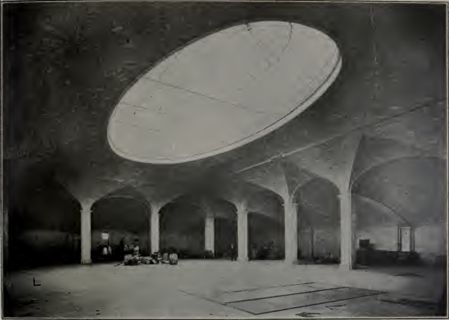
THE HUGE GUASTAVINO VAULT ON THE TOP FLOOR OF TIFFANY & CO.'S BUILDING.
