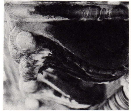
Dirt buildup on a cornice
