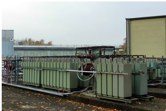
Figure 57 One of several energy storage power film capacitor banks, for magnetic field generation at the Hadron-Electron Ring Accelerator (HERA a ), located on the DESY b site in Hamburg c
