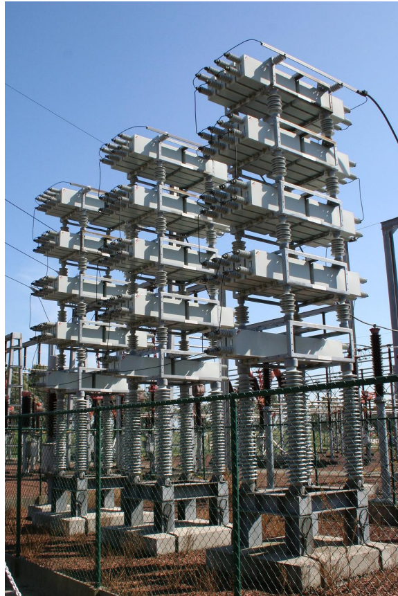
Figure 58 75MVAR substation capacitor bank at 150kV
