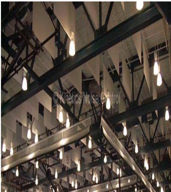
Noise Control Baffles (fiberglass)
