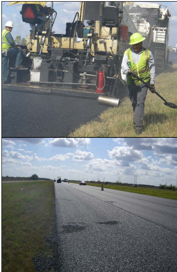
Figure 5. MTV Paving Operation (upper photo) and Areas in the Mat where Cold Chunks Required Removal and Patching (lower photo) on US 288 in the Houston District.
