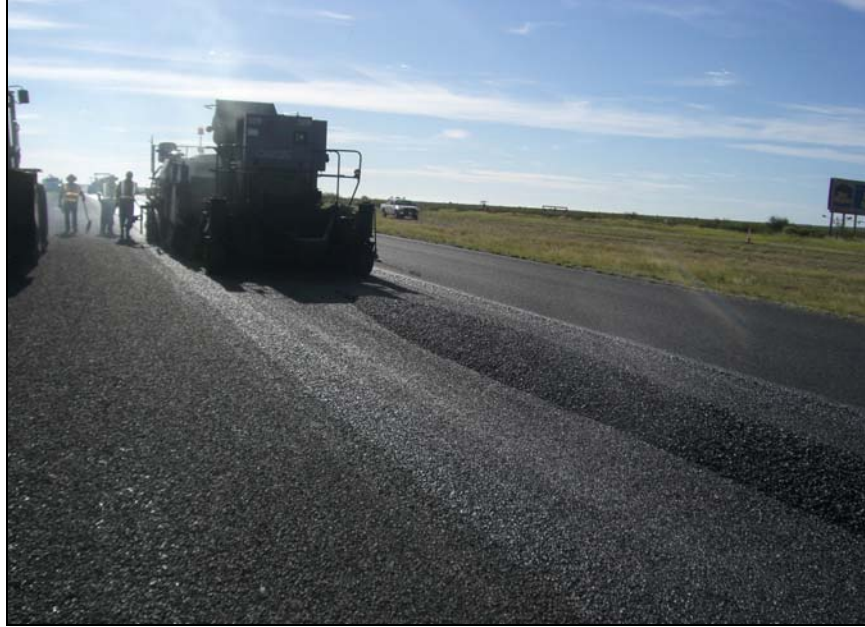
Figure 3. Application of PFC on Tacked, Newly Seal Coated Surface of IH 10 in Odessa District.
