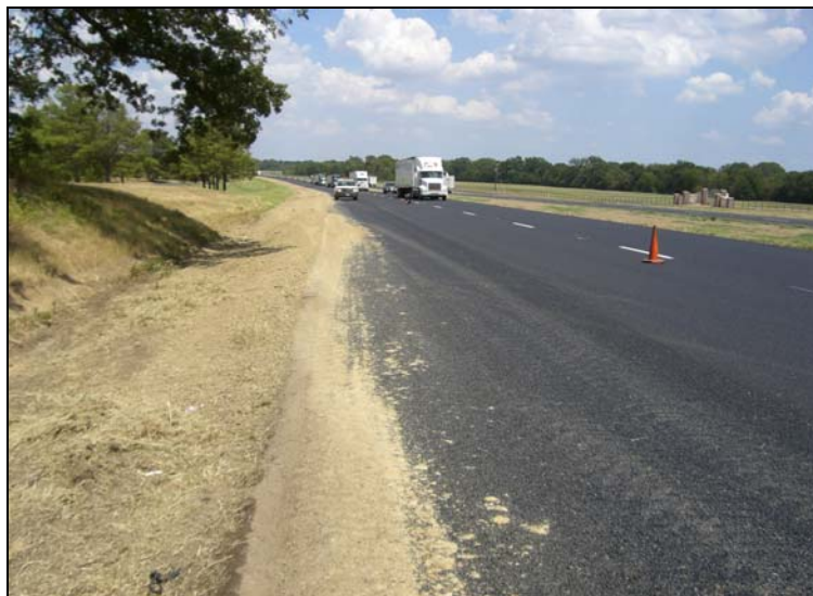
Figure 2. Edge Clearing that Can Cause Clogging of PFC Restricting Lateral Water Flow.
