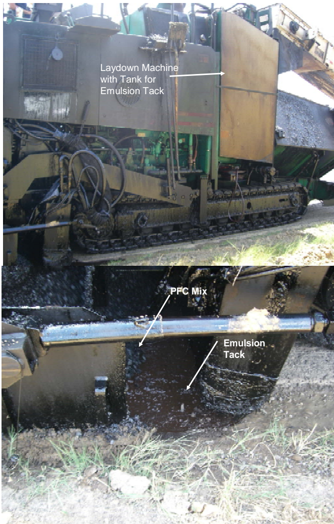
Figure 4. Laydown Machine with Tank for Applying Tack on IH-30 in the Paris District.
