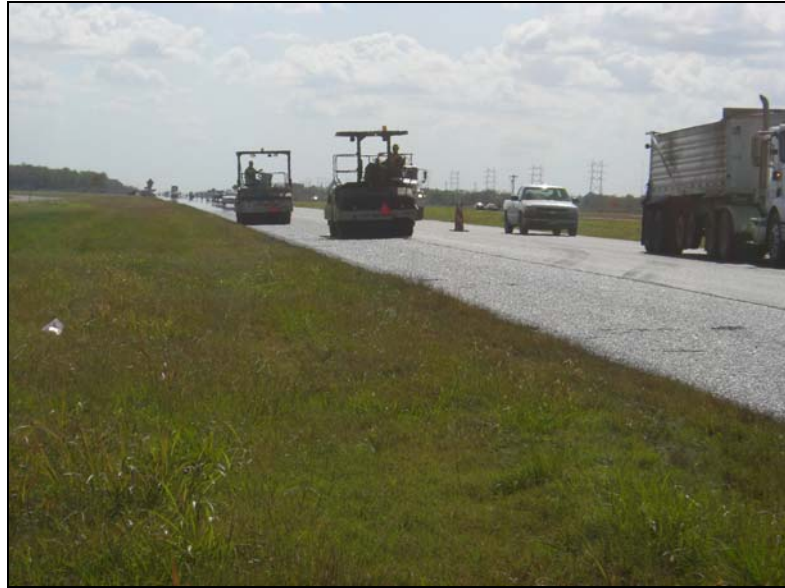
Figure 11. A Single Roller Pass as Allowed in the Houston District (No Roller Back Up Allowed).
