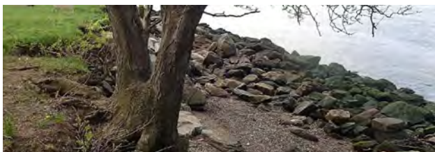
Understand shoreline conditions: Eroded riprap
