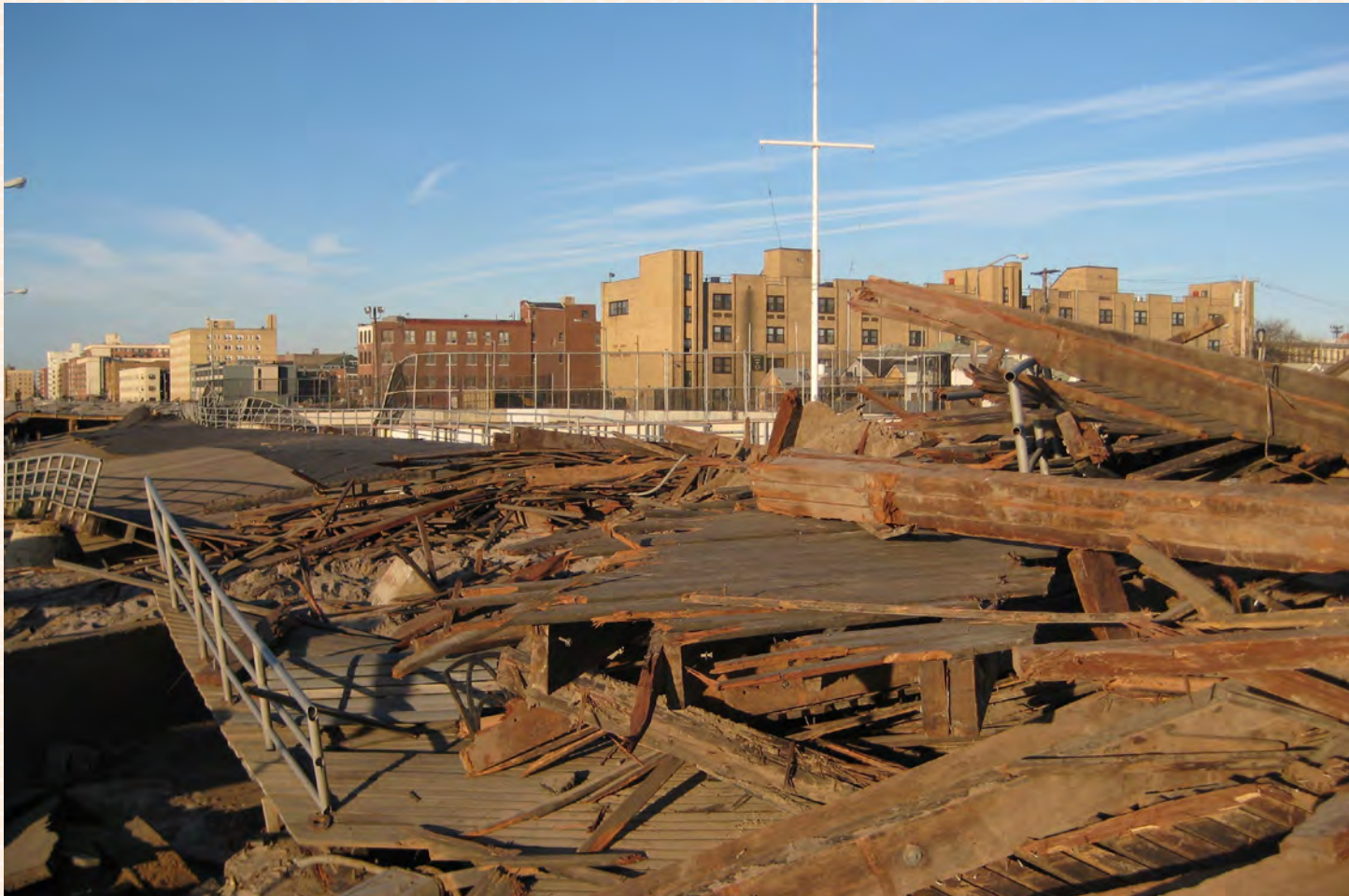
Damaged boardwalk at Rockaway Beach, Queens
