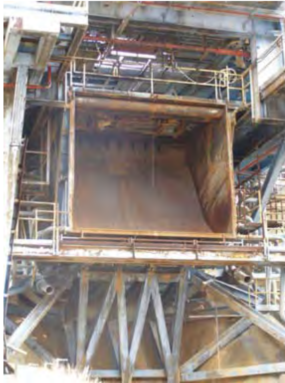
Photo 4.7. Alfa I Test Stand, flame deflector, camera facing northeast. (Source: Archaeological Consultants, Inc., 2007.)
