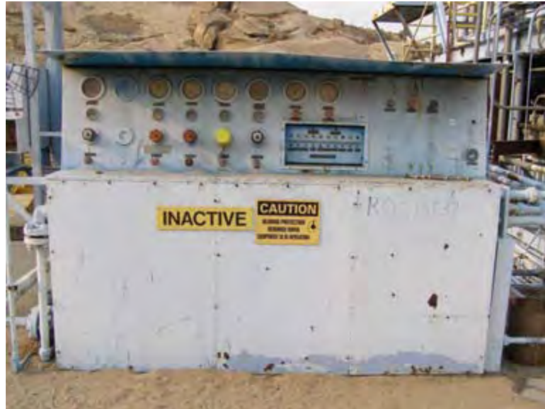
Photo 4.9. Alfa I Test Stand, Pneumatic Gauge Panel, camera facing south. (Source: Archaeological Consultants, Inc., 2007.)
