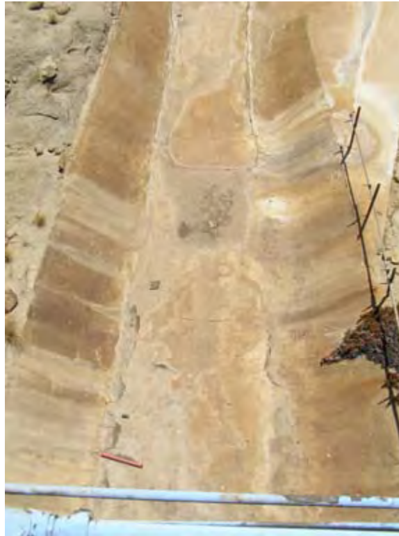
Photo 4.12. Alfa III Test Stand, gunite channel, camera facing south. (Source: Archaeological Consultants, Inc., 2007.)
