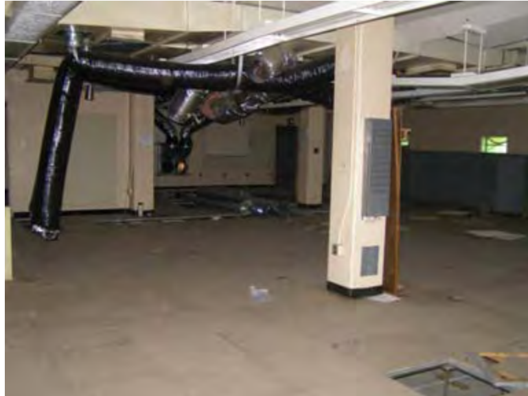
Photo 4.59. Coca Control House, Test Operations Room, camera facing northeast. (Source: Archaeological Consultants, Inc., 2007.)
