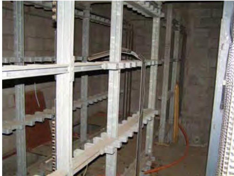
Photo 4.60. Coca Control House, stage terminal room, camera facing northeast. (Source: Archaeological Consultants, Inc., 2007.)
