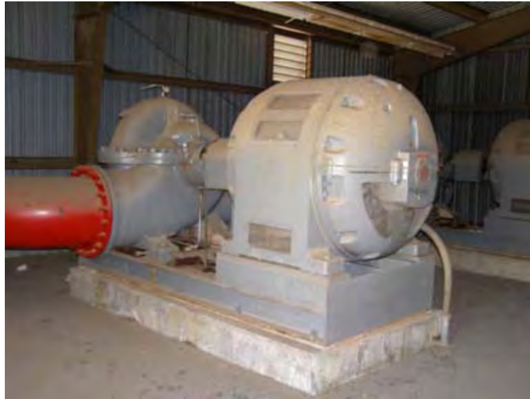
Photo 4.48. Pump detail, camera facing northeast. (Source: Archaeological Consultants, Inc., 2007.)
