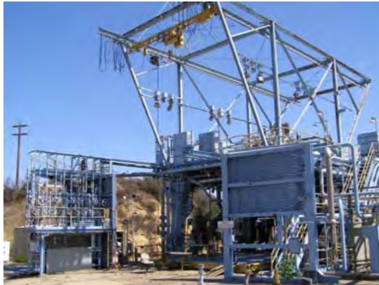
Photo 4.26. Bravo I Test Stand, west and south elevations. (Source: Archaeological Consultants, Inc., 2007.)
