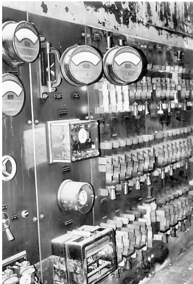
Figure 4 - The “totalizing” panel of the dc switchboard.
