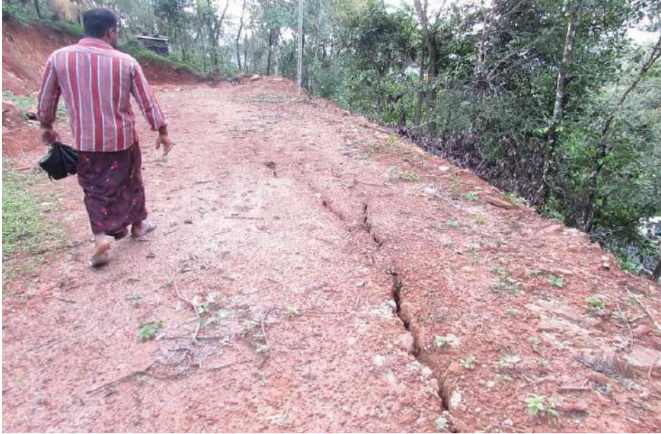
Crown cracks developed in Valad Kunnathumal road
