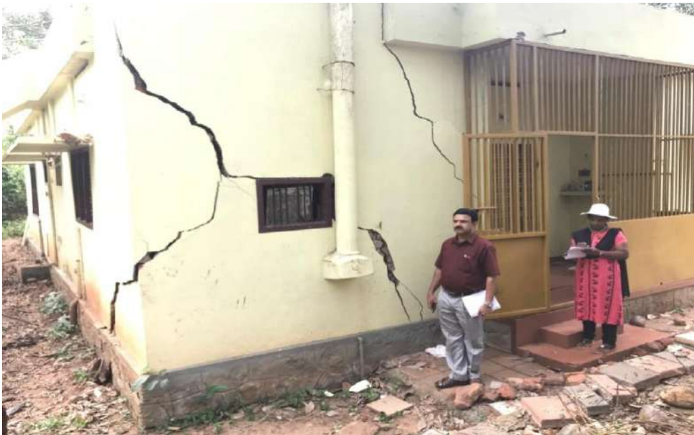
Cracks on buildings due to landslide in Pananchery panchayat
