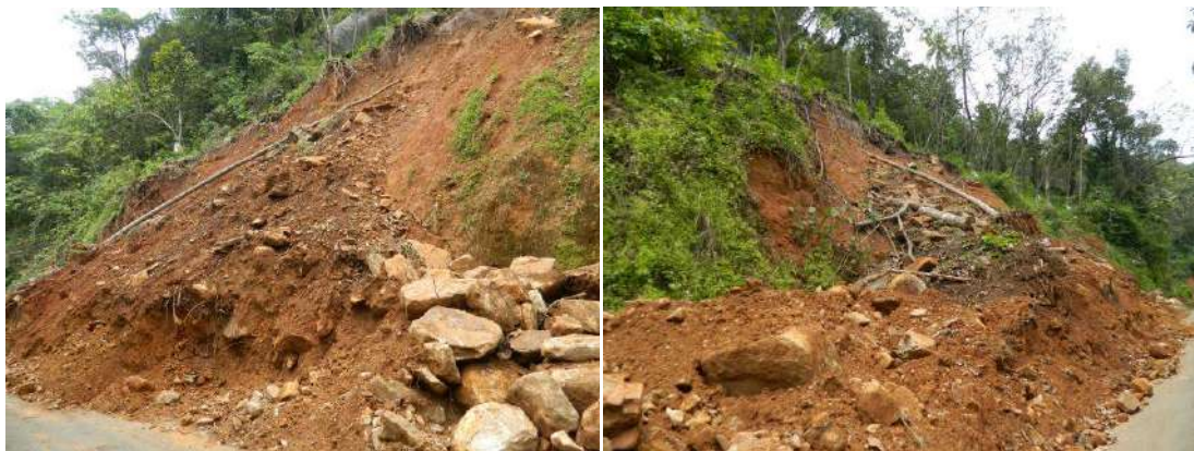
Land slide affected Area in Kanjirapilly Taluk
