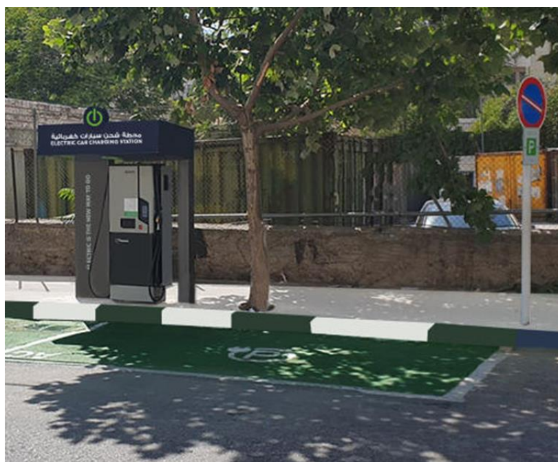
Figure 6.1 Electric vehicle fast charge station in Hebron
