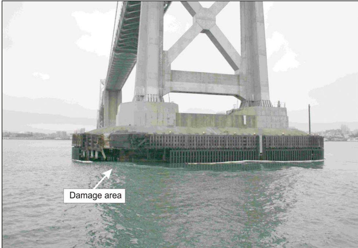
Figure 5. Damaged fendering system at the base of the Bay Bridge Delta tower.
