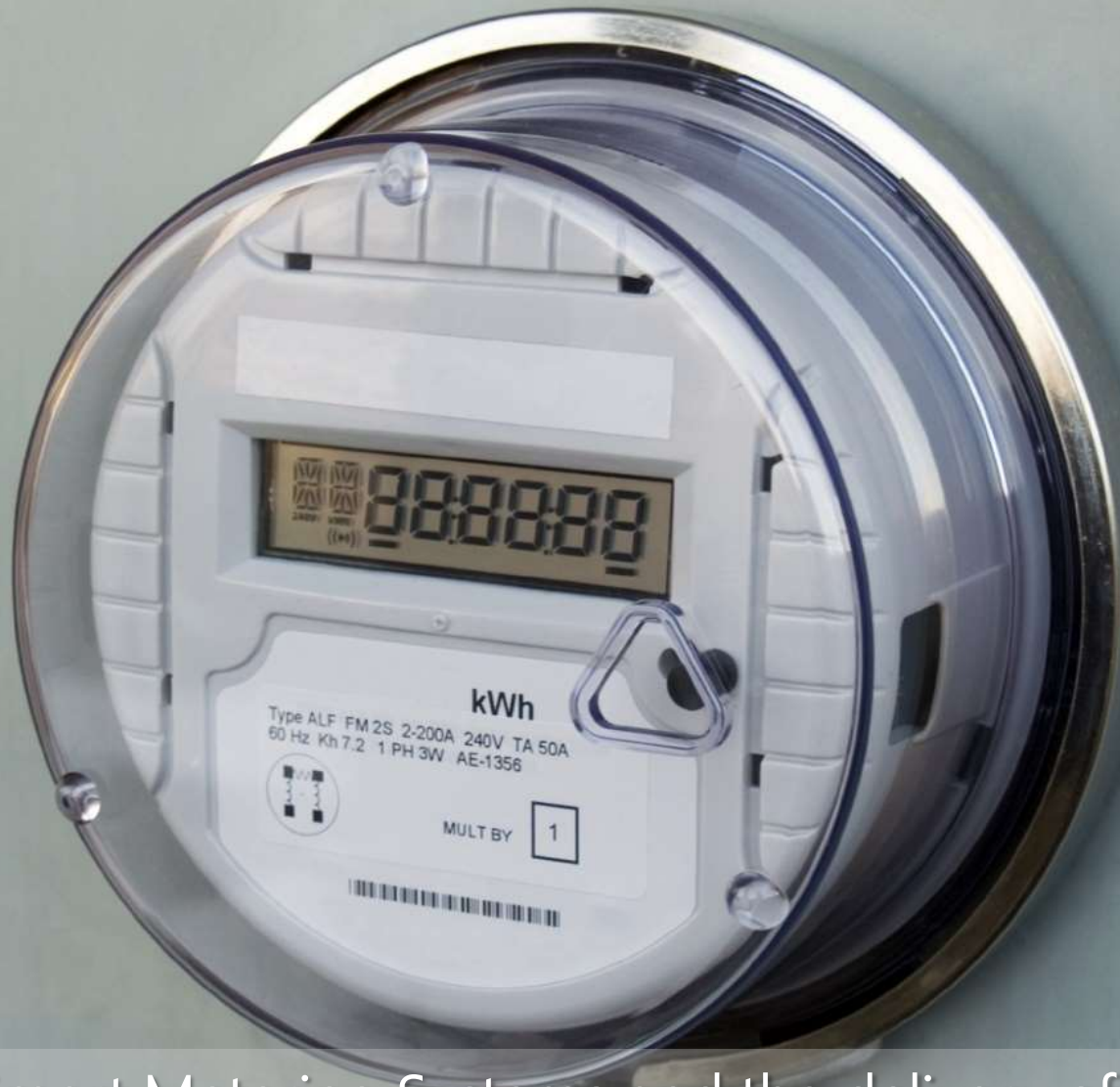
HSMs secure Smart Metering Systems and the delivery of Meter messages in our homes to Head End Utility systems
