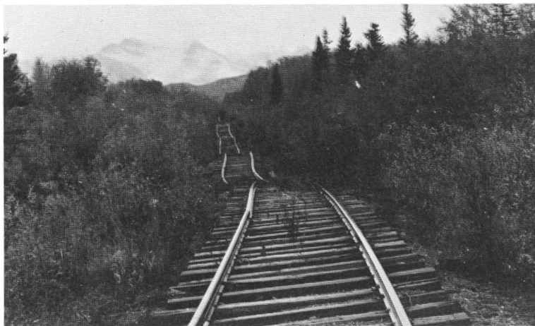
Ground subsidence along the abandoned Copper River Railroad.
