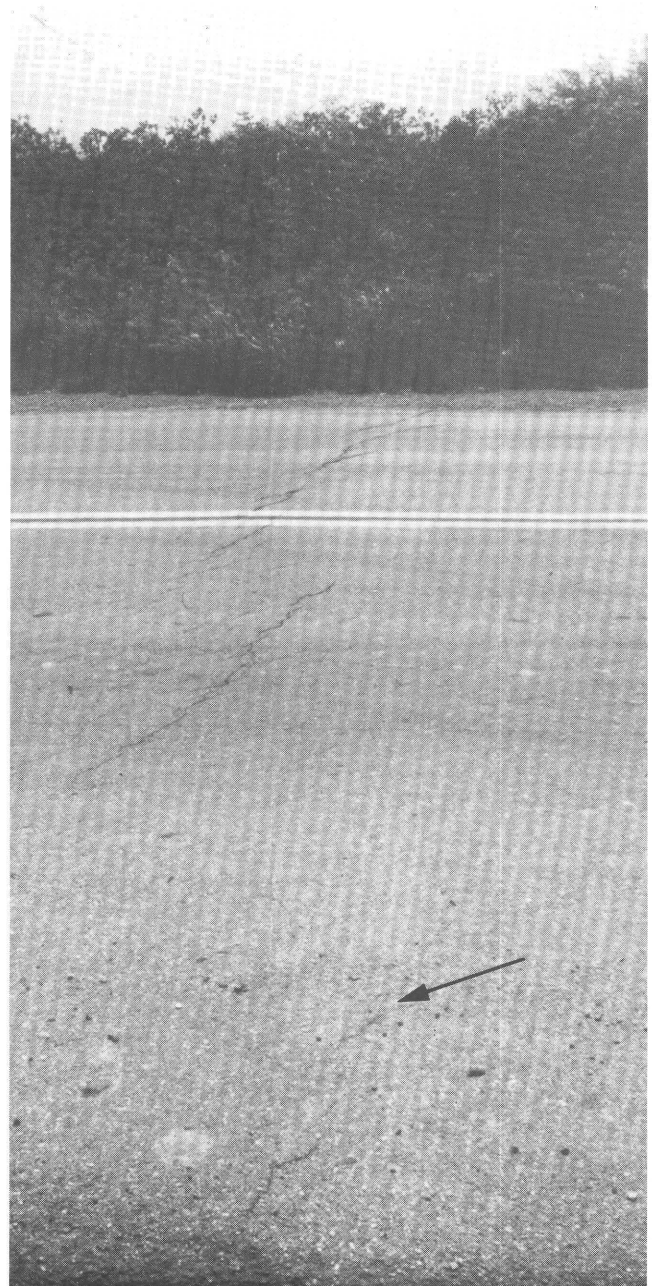
Figure 13.6. Calaveras fault trace at Shore Road. Station SHR1 is in shoulder in upper left center. Arrow denotes hairline crack extending from dirt shoulder into roadway. View southeastward.
