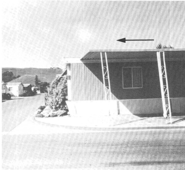
Figure 11.11. Partly collapsed mobile home in Madrone Mobile Home Estates (loc. 7, fig. 11.2). Carport supports were perpendicular to ground before the earthquake. Arrow shows direction of motion. View westward.
