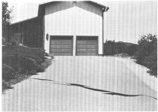
Figure 10.3. Conspicuous fissure in a driveway near crest of hill above house shown in figure 10.1. Fissure was caused by local ground displacement, probably an incipient slope failure, but had no direct influence on damage to houses in the area.
