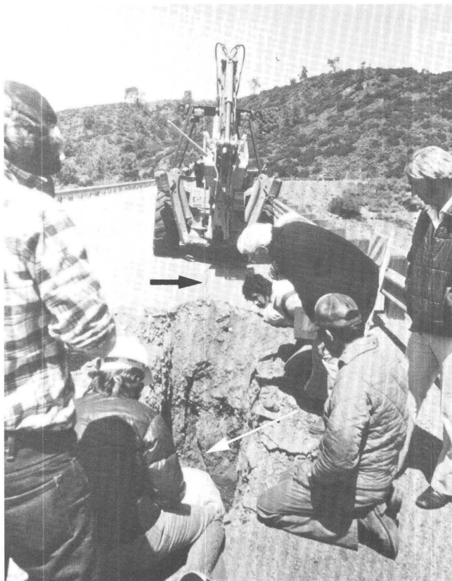
Figure 11.20. Soil-pit-type trench through crest of the Anderson Dam (loc. 22, fig. 11.7). Crack in pavement, visible in north vertical trenchwall, appears to curve outward toward upstream face of dam, to right near bottom of excavation. Arrows point to cracks at surface and at depth. View north-northwestward.
