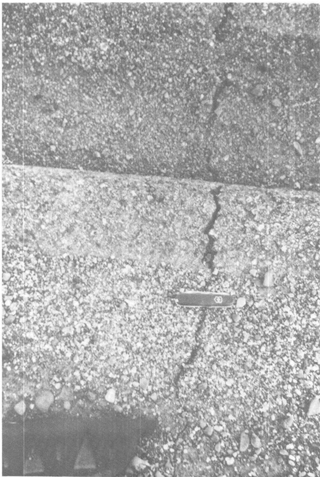
Figure 7.3. Calaveras fault at California Highway 152 (Pacheco Pass Road) on April 25, 1984. Crack in darker upper part of photograph is in asphalt of the road. Crack in lighter middle part above knife is in road curb, which is offset about 1 cm right laterally. Crack beneath knife in foreground, in dirt alongside the road, also shows right-lateral offset.
