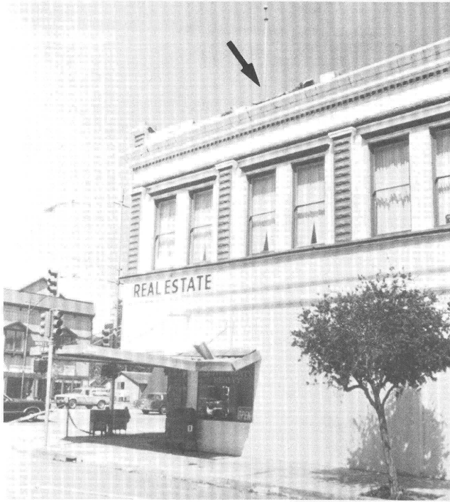
Figure 11.3. The 1905 or South Coast Realty Building (loc. 1, fig. 11.2). Tumbled part of roof cornice fell to north (arrow). Note partly collapsed awning near left corner of building that was struck by a heavy object, possibly a block from the cornice. View northwestward.
