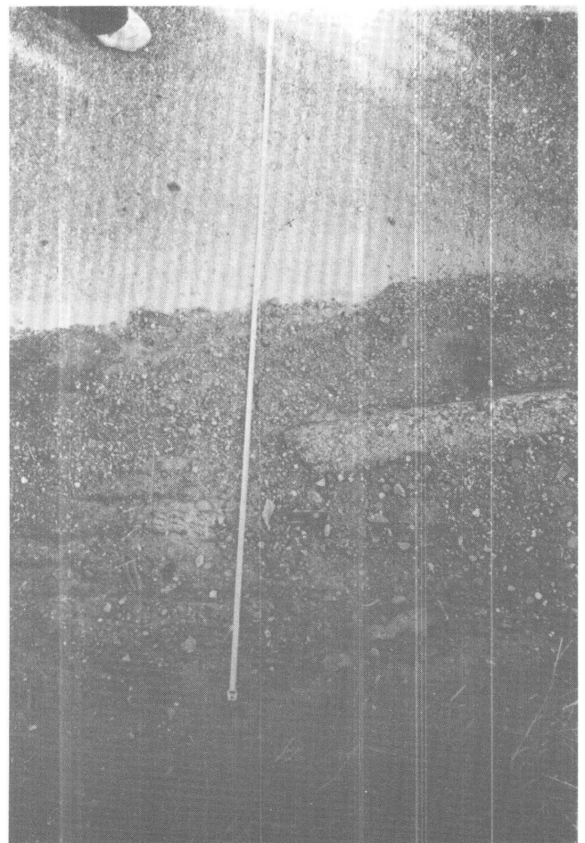
Figure 7.4. Calaveras fault at California Highway 152 (Pacheco Pass Road) on April 25, 1984. Crack is northeast of the one in figure 7.3. Crack in lighter upper part of photograph to right of tape is in asphalt. Crack in darker lower part is in dirt and runs from underneath knife downward and underneath tape, about 1.5 knife lengths from end of tape.
