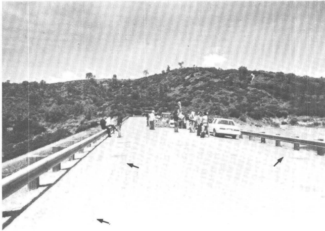
Figure 11.19. Longitudinal cracks developed along crest of the Anderson Dam (loc. 22, fig. 11.7). Trench used to investigate behavior of cracks at depth was excavated parallel to longitudinal upstream crack at right center. Arrows point to crack sets. Upstream is to right. View north-northwestward.
