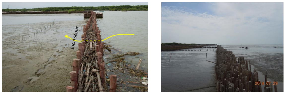
Figure 7.2 Left panel: “classical” permeable structure with brushwood; right panel: bamboo fence (both deployments in Indonesia)
