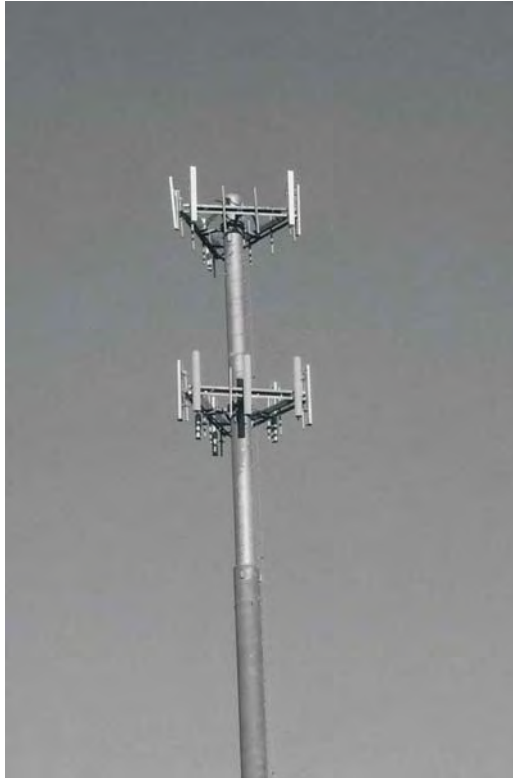
Figure 2.14 A typical cellular/PCS antenna system; actually, two collocated systems are shown. Note the three antenna elements per sector, generally two receive antennas and one transmit antenna.
