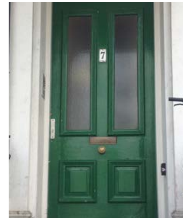
Typical Victorian four panelled door with glazed panes used for Italianate houses
