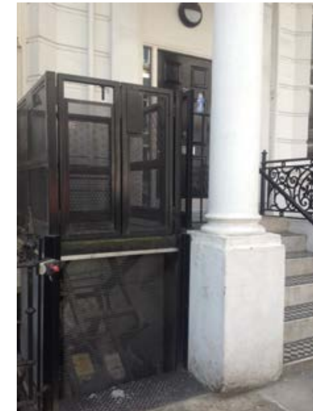
Wheelchair lift at hotel
