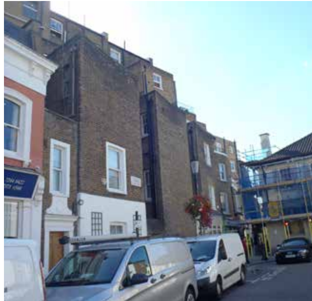
Gaps between closet wings rear of nos. 9-13 (odd) Hogarth Rd
