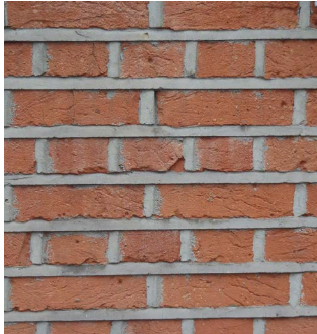
Heavy weather struck cement pointing
