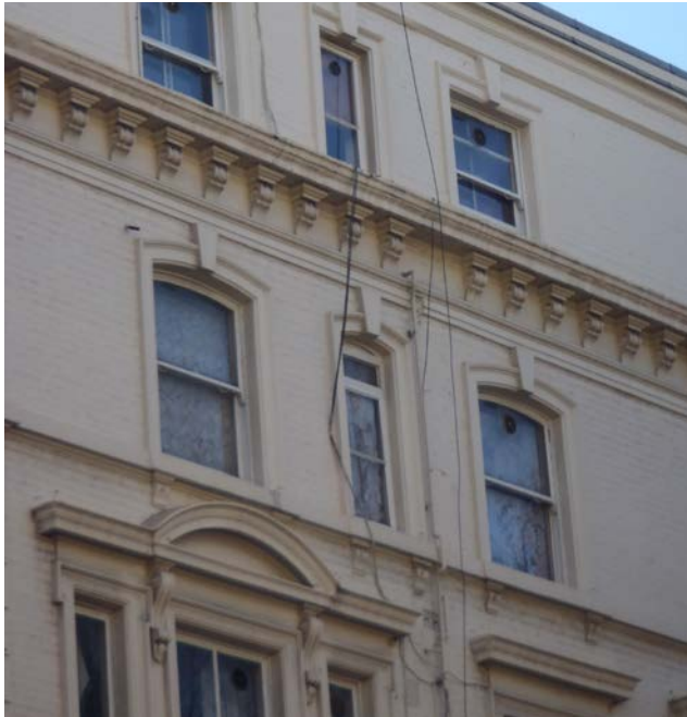
Cables attached to building
