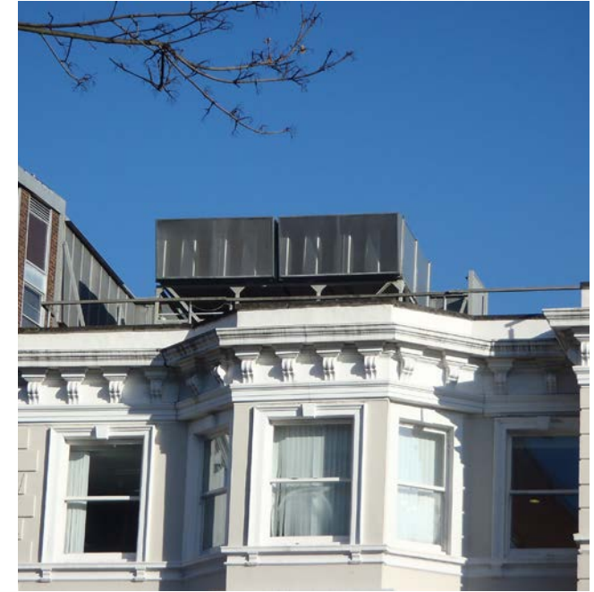
Plant to roof
