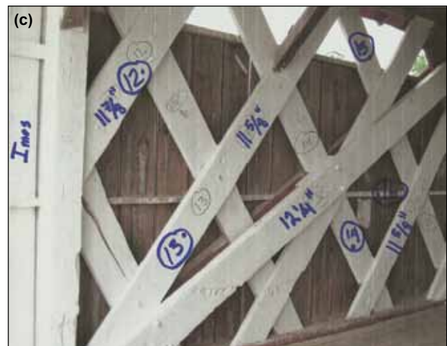
Figure 39. Locations on the Imes Bridge where comparison measurements were taken using traditional tape measures and extracted from the digital point clouds created from the laser scanning process.
