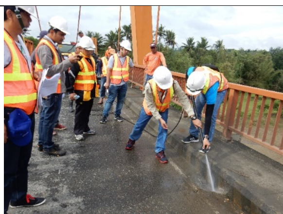
3 rd OJT on Routine Maintenance Manual Mar. 02, 2017 Cleaning of Drainage using High Pressure Water Blaster at RO-II Magapit Bridge
