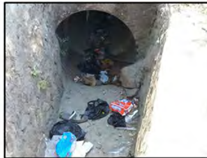
Waste inside drainage system
