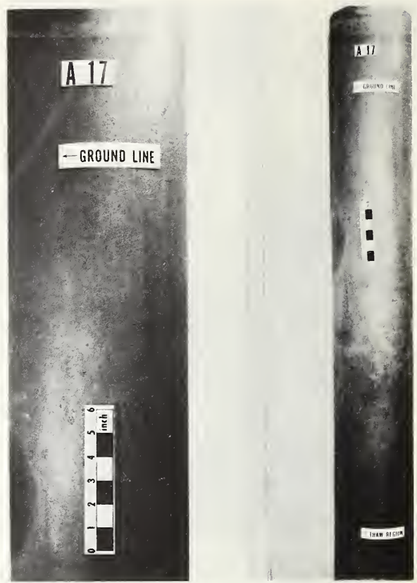
FIGURE 4 - Conditions of sections of pipe pile A17 exposed above the ground line and in the active (thaw) region. Final inspections of these sections were made in the laboratory.
