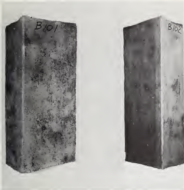
FIGURE 6. Sandblasted sections of Z-type sheet piling cut from two different locations in the Vicksburg Floodwall after exposure for 7 years.
