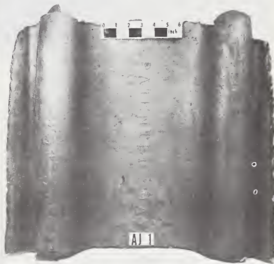
FIGURE 3 — Section of steel sheet-pile pulled from an engineer's slip on the Niagara River at Buffalo, N. Y., after exposure for 36 years. The section was exposed about 8 ft below the ground line in the water table zone.
