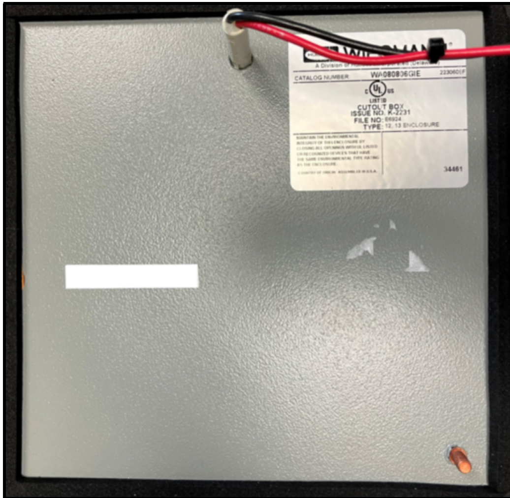
Figure 3.4: Interior door view of the interface box.
