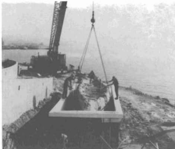
19) Within a record ten days a reinforced concrete conservation pool was built by the museum. The boat was then gently placed inside the pool. Courtesy Israel Antiquities Authority. Photo: D. Syon (Friedman).
