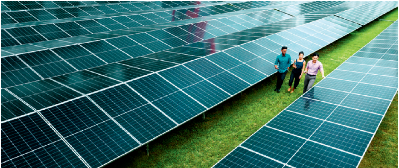
Photovoltaic panels at our Hougang Telephone Exchange generate approximately 0.77GWh of energy annually.
