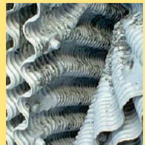
Deposit may be biofouling. Further investigation is required
