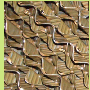
Staining and not a deposit
