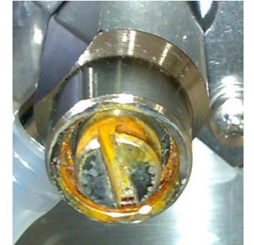
Corrosion of Ni-plated brass drain valve of the chiller
