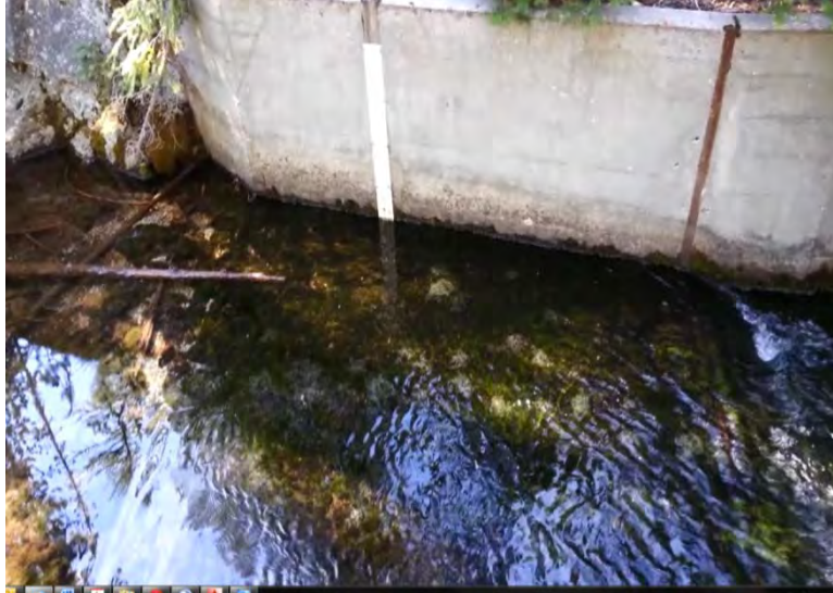
Photo 39 - Nada Lake Parshall Flume, View from South Looking North (Flow Left-Right)
