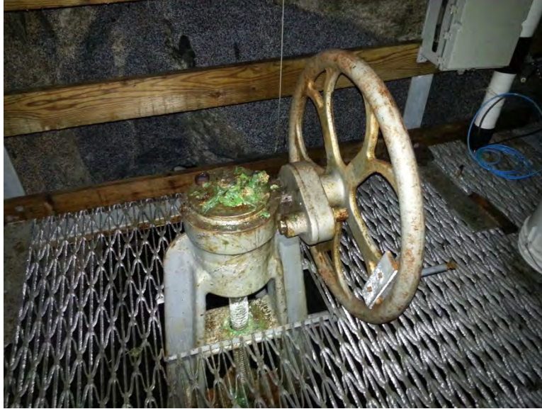
Photo 31 - Upper Snow Lake Outlet Works - Gate Valve Actuator
