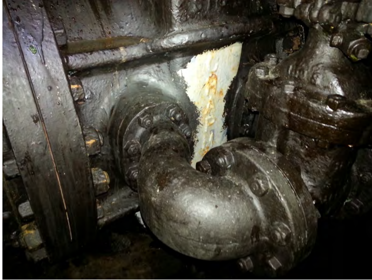
Photo 33 - Upper Snow Lake Outlet Works - Gate Valve Pressure Equalization Bleed-Bypass Valve
