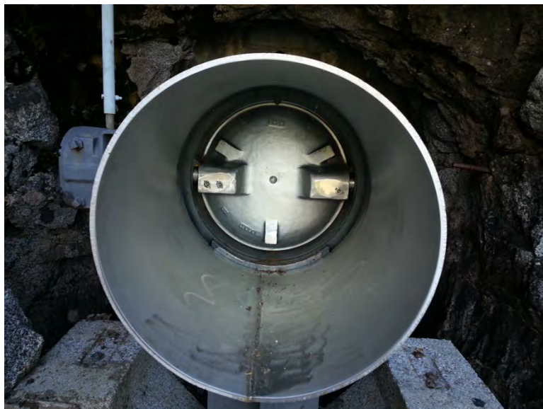
Photo 30 - Upper Snow Lake Outlet Works - Butterfly Valve
