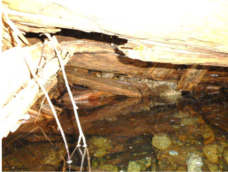
Photo 10 – Lower Klonaqua Outlet Works Tunnel - Collapsed (View from Channel Downstream)
