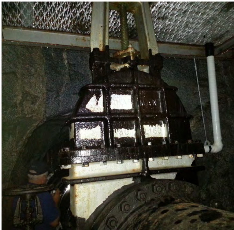
Photo 32 - Upper Snow Lake Outlet Works - Gate Valve, View looking Towards Snow Lake
