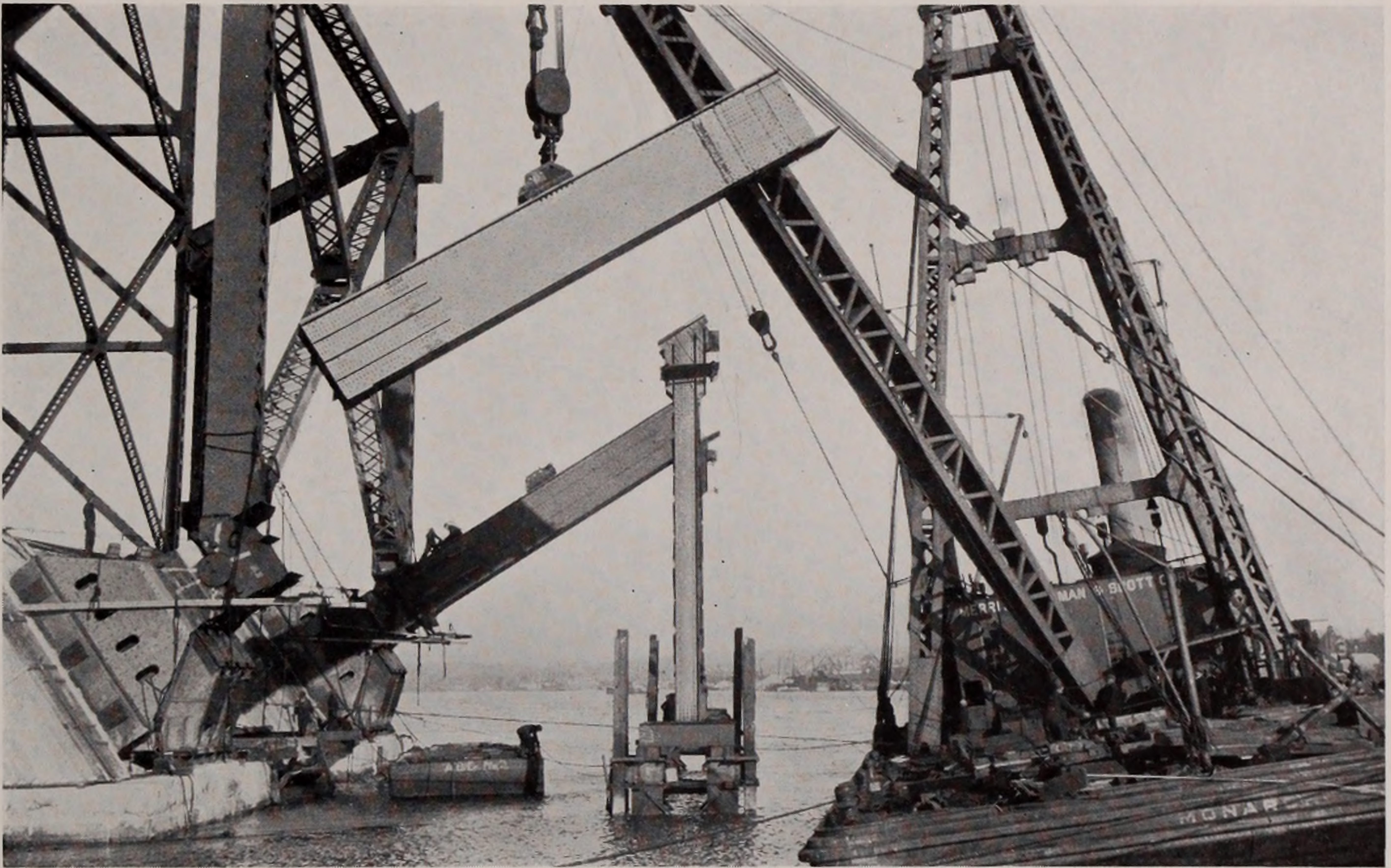
ERECTING FIRST PANEL BY DERRICK BOAT, BAYONNE SECTION OF THE ARCH. APRIL 9, 1930
