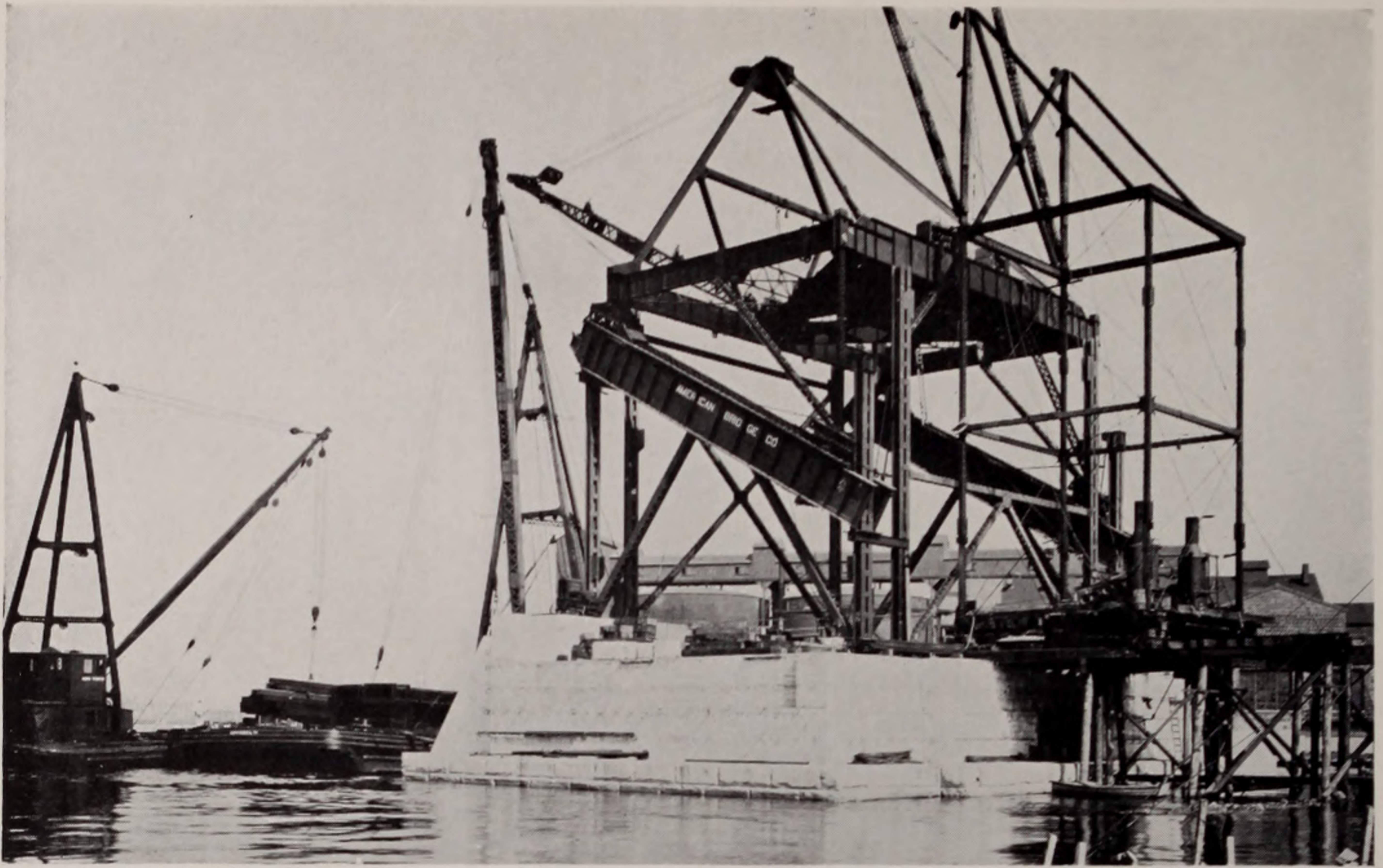
ASSEMBLING TRAVELER AT THE PORT RICHMOND ABUTMENT FOR ERECTION OF THE SOUTH SECTION OF THE ARCH. SEPTEMBER 25, 1929
