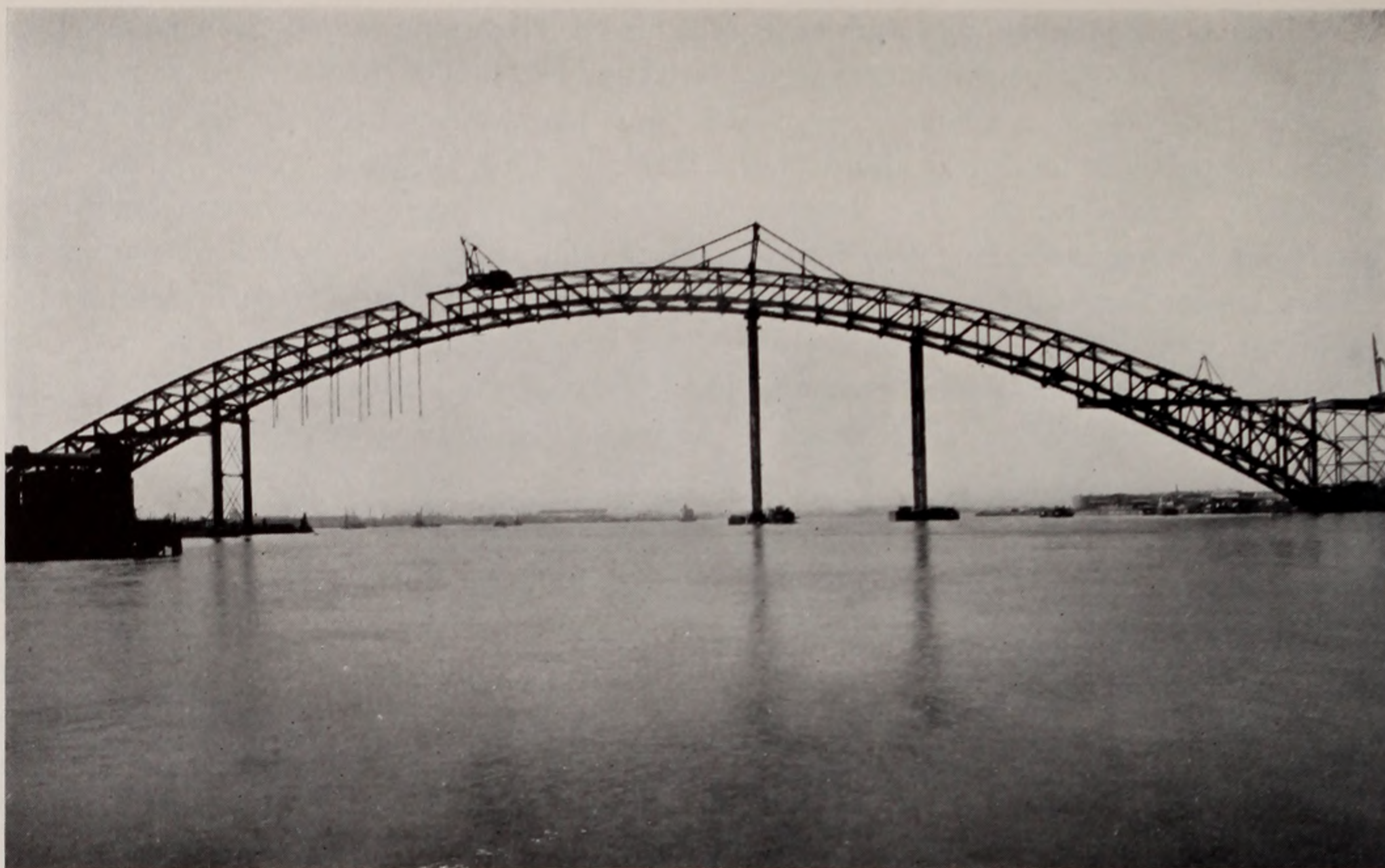
KILL VAN KULL ARCH READY FOR CLOSING OPERATION, BAYONNE ABUTMENT AT RIGHT. OCTOBER 2, 1930
