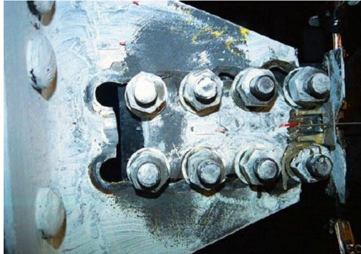
Figure 6.24: Failure surface of block shear/tearing ( https://m2ukblog.wordpress.com/2016/05/28/block-shear-failure-in-tension-members/ )
