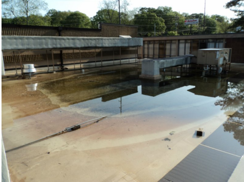
Figure 2.15: Ponding on roof
