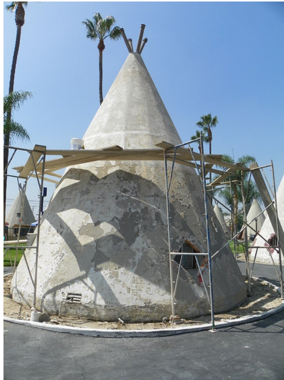
Figure 6.4: A missed opportunity for sharing preservation efforts. This picture was taken by a tourist during one of the major renovations at Number 7. Courtesy of Flickr user ewaldmire, https://flic.kr/p/abTx8i .
