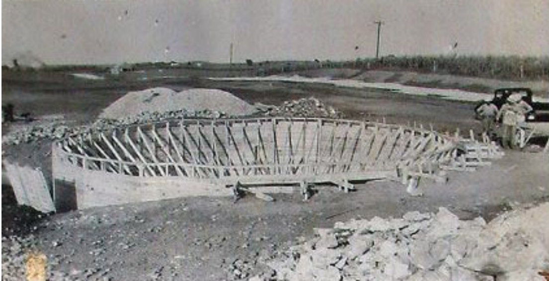
Figure 5.2: The basement during Village Number 2's construction. Courtesy of Flickr user Wiley Brewer, https://flic.kr/p/8aA7Av .
