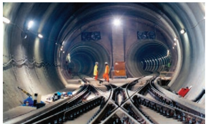
● Heathrow Express Triumph in partnering following the 1994 collapse
