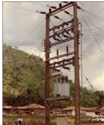
● Electricity supply Power lines, Kenya
