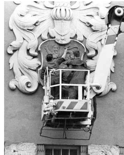
The restoration of the Tallinn coat of arms on the Estonian Drama Theatre. Tallinn's oldest symbol had been plastered over due to its similarity to the coat of arms of the Republic of Estonia.
