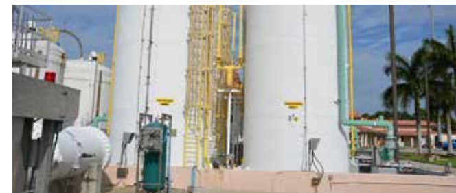
| WTP 9 Sodium Hypochlorite Tanks |
