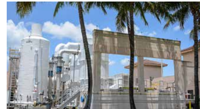
| WTP 3 Clearwell #1 Odor Control System |
