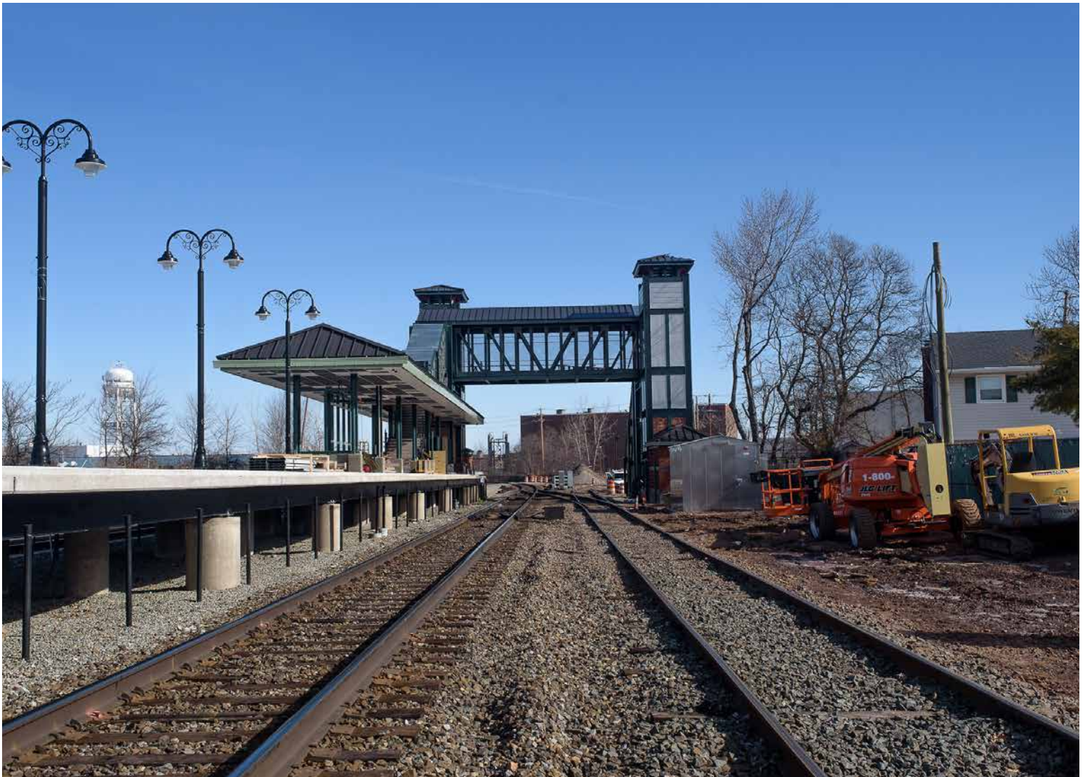
Work is progressing on the new Wesmont Station on the Bergen County Line.
