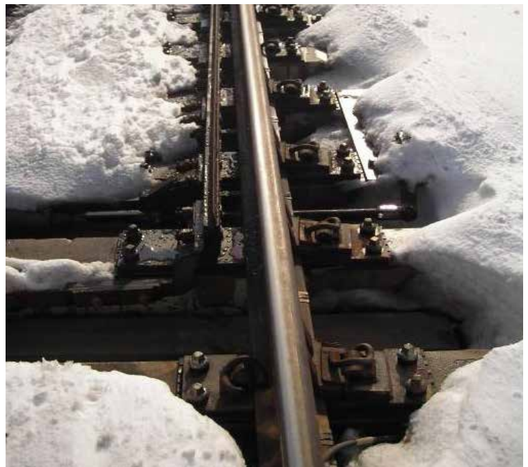
New energy-efficient switch heaters, which keep train switches free of snow and ice, conserve electricity.
