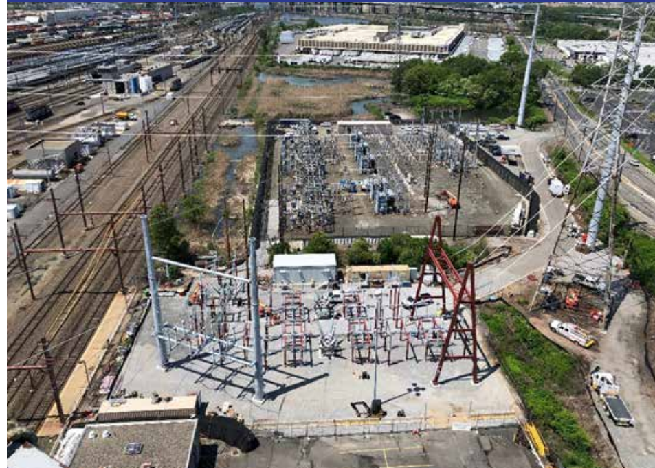
EXISTING: Mason Substation
