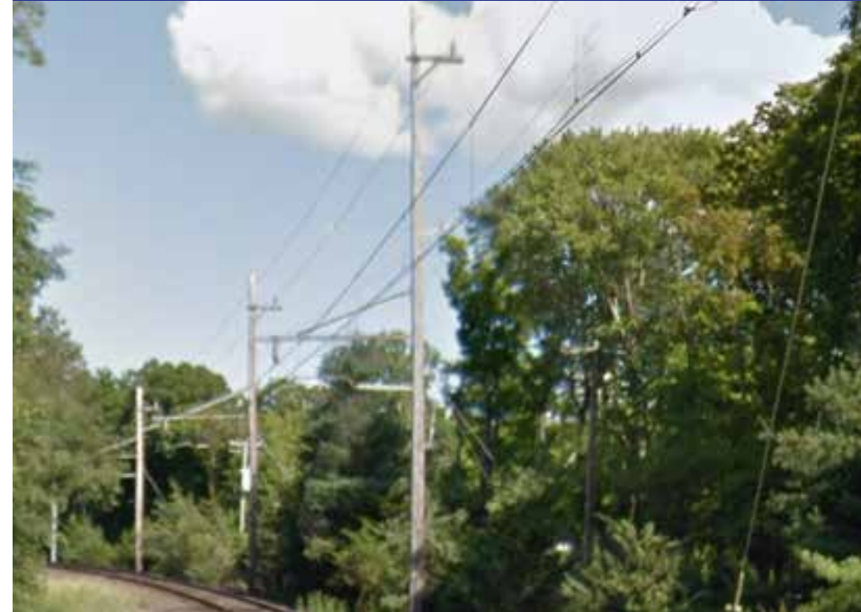
EXISTING: Wood Poles
