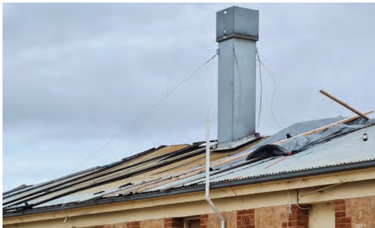
The McCoy Street building that Waikerie woman Rosie Reiss claims is unsafe.
