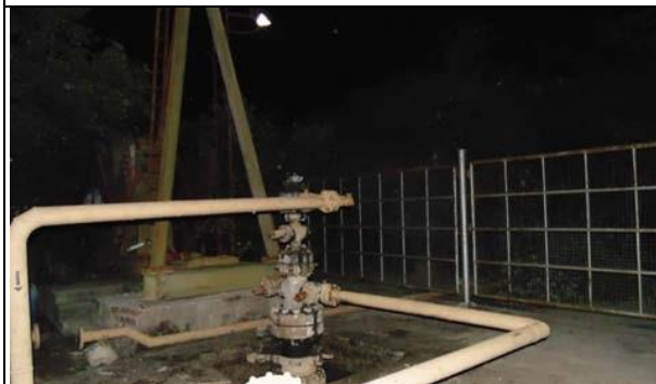
Abandoned oil well near Mattur, Needamangalam, Thiruvarur (Location: 10°50'40.70"N 79°26'28.14"E)
