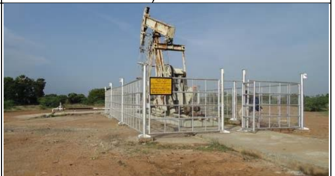
Sucken Rod Pump mechanized oil well near Greater Kovil Kalappal, Thiruvapur District (Location: 10°34'03.21"N 79°31'50.18"E)
