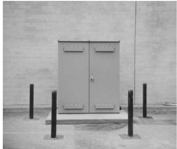
New Service Entrance Section with Meter
