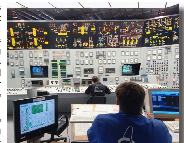
VVER Control Room Novovoronezh NPP, Russia [6]
