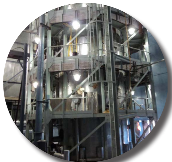
Hydrogen recombiner test facility for future improvement for HWR (Courtesy of NPCIL)
