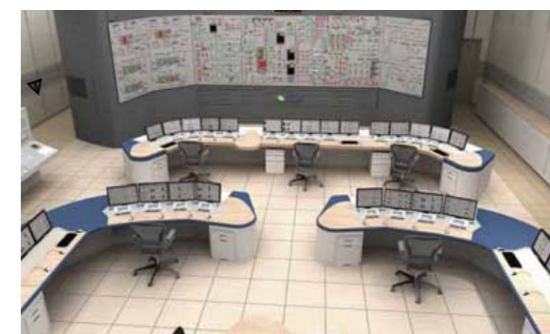
AP1400 Main Control Room (KEPCO)
