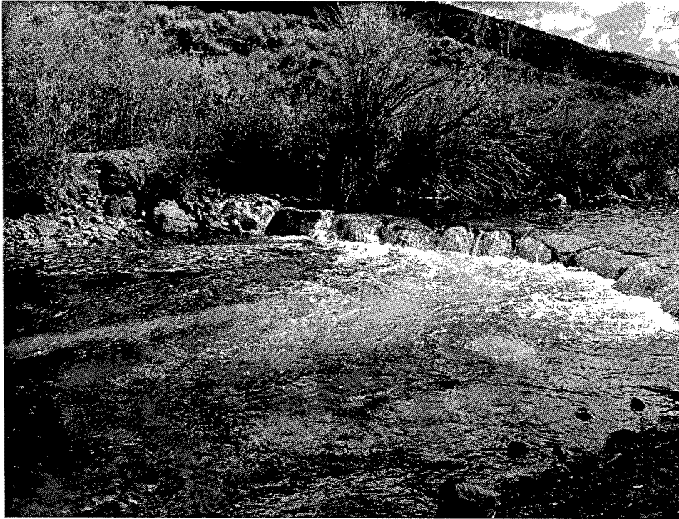
Figure 8. Low-head stone weir on the North Fork of the White River, Colorado
