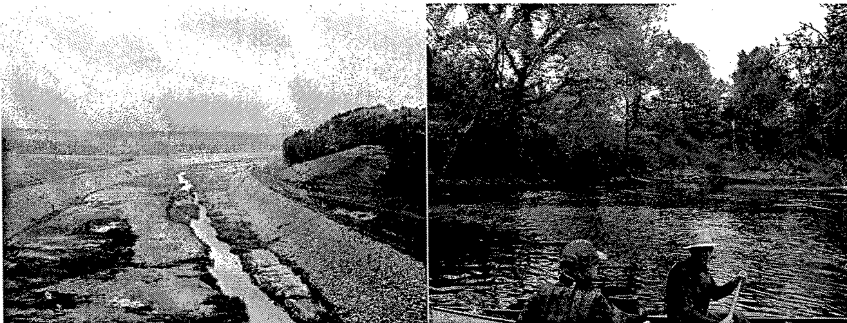
Figure 3. Common problems include setting the riprap elevation higher than needed and not extending the protection far enough downstream
