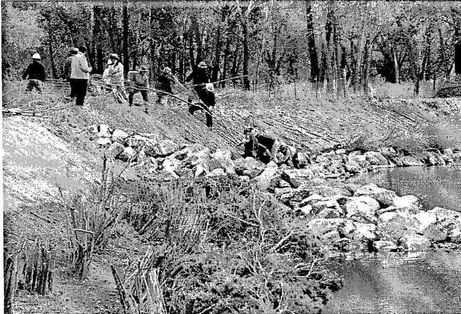
Figure 4. Incorporating irregular alignments, features such as spurs, and other habitat measures into a revetment can significantly improve habitat benefits
