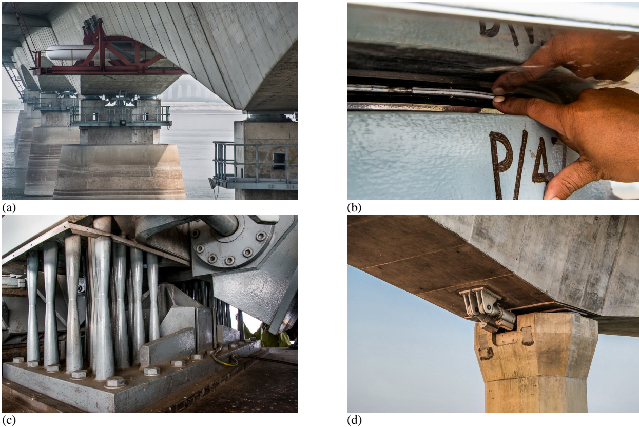
Figure 23. Bearings and Joints in (a) Bangabandhu Bridge, (b) Pot bearings of Bangabandhu Bridge, (c) Pintels in Bangabandhu Bridge, (d) Shock Transmission Units in the Lalon Shah Bridge.
