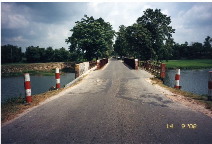
Figure 7. Composite steel bridge fabricated by Miyaji Iron Works Co., Tokyo, Japan in 1958. Photo courtesy: Mr. I.A. Khan, OBE, Formerly Rendel Palmer & Tritton in Dhaka, Bangladesh.
