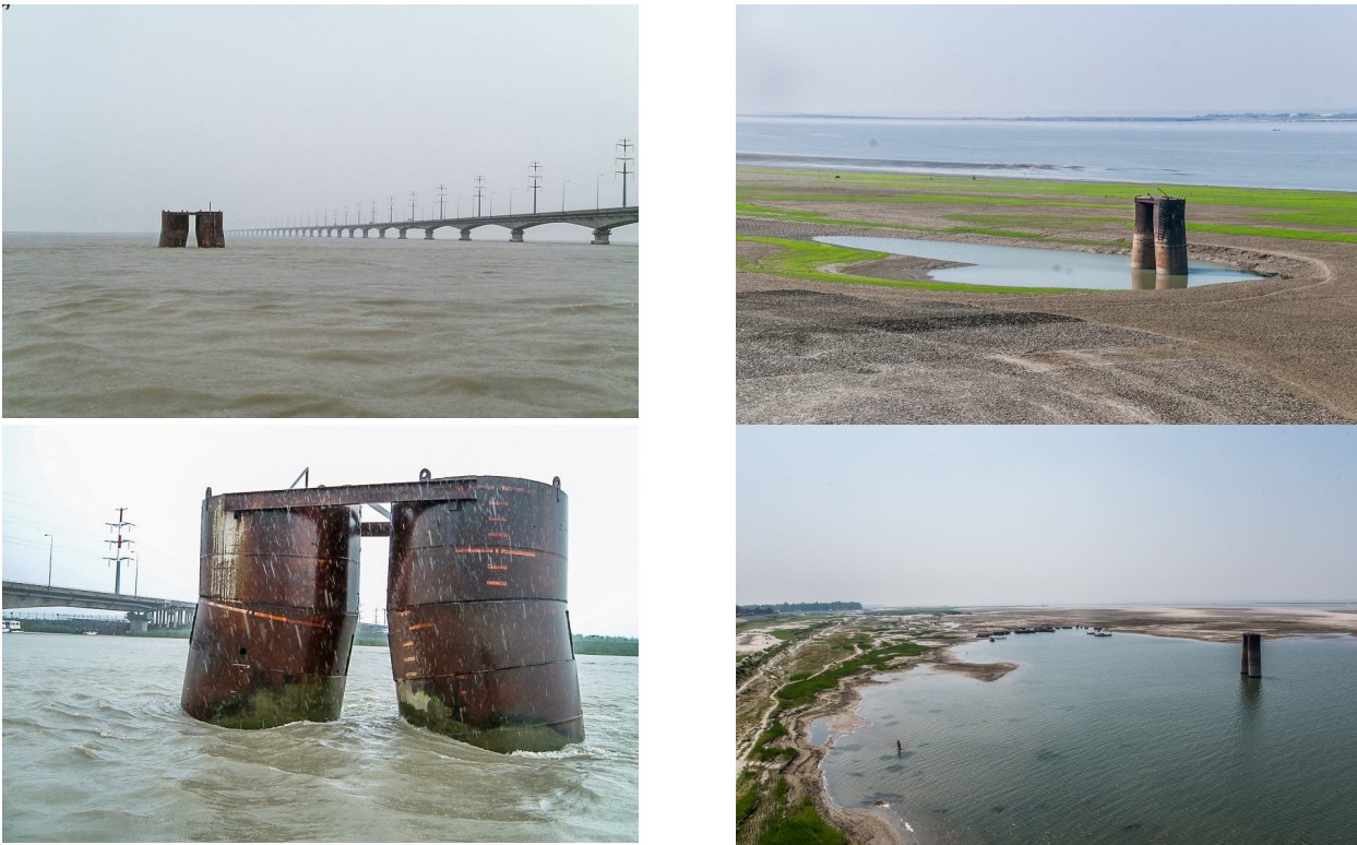
Figure 17. Water levels at Bangabandhu Jamuna Bridge over different seasons as seen around the inclined concrete filled steel tubes driven as test piles during construction of the bridge. Local scour around the test piles are visible in dry season photos.
