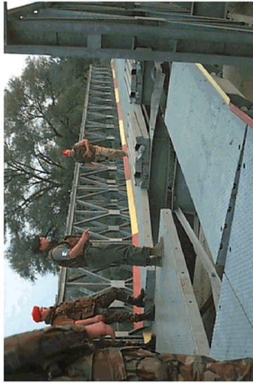
P13103_1.JPG 021915JUL96 BQ68055480 VICINITY OF USORA BRIDGE DAMAGED DECKING DC-40
