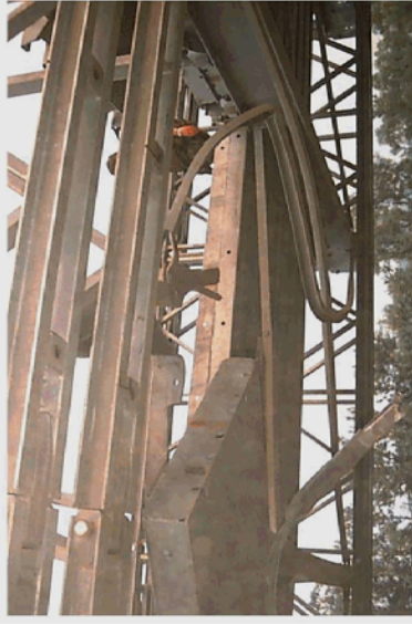
P13103_3.JPG 021915JUL96 BQ68055480 VICINITY OF USORA BRIDGE VIEW FROM UNDER BRIDGE LOOKING UP DC-40
